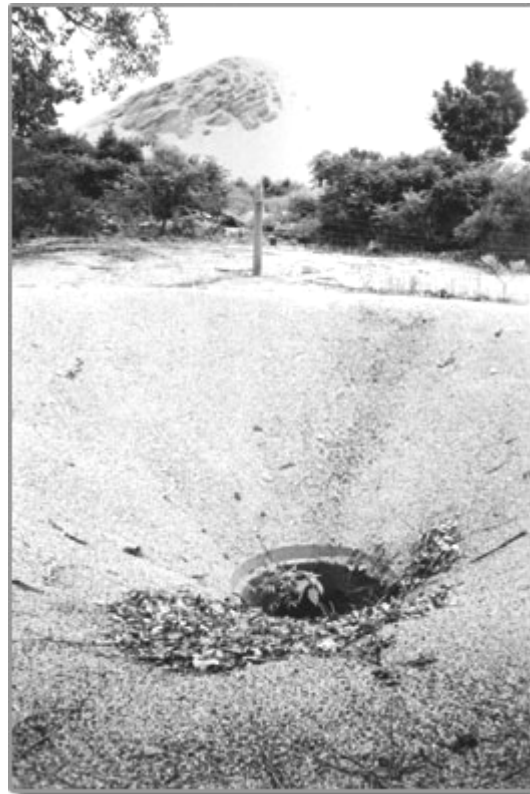
Another open mine shaft in Picher, also not fenced off, is not on any list of remediation projects. In the background is a large chat pile.
